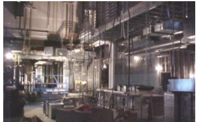
Mechanical Mezzanine, Area B – Impressive!
