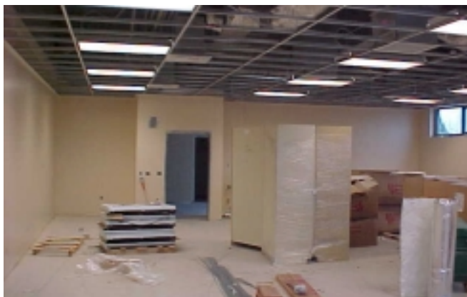
12/21/04 - Permanent lighting activated in the Weight Rm., Area A.
