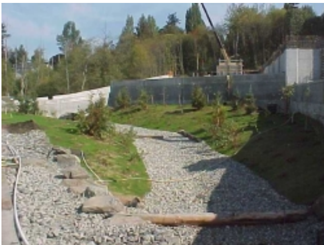
View of the south end of the new Hall Creek stream channel.
