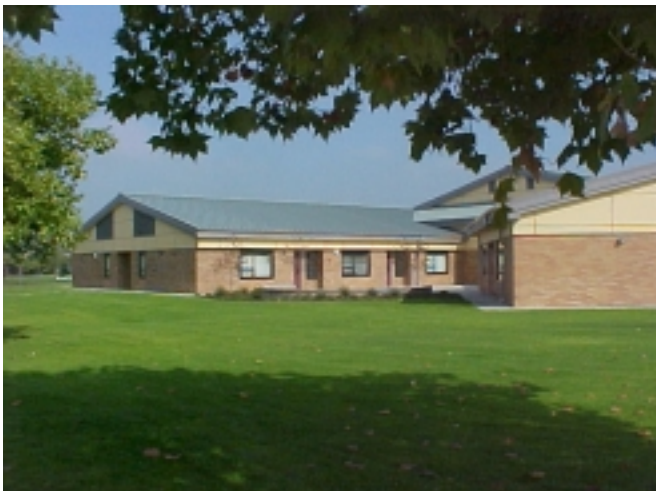
Phase 1 & 2 ('A' Wing Remodel) nearing completion & the end to another beautiful day at the LaVenture Site.
