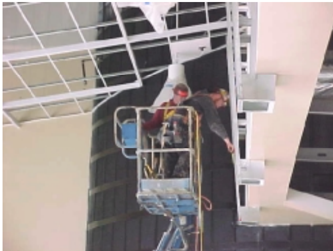
03-22-05 - Kidder Anderson & Eric Dysert in manlift at Commons installing MDF wall panels.
