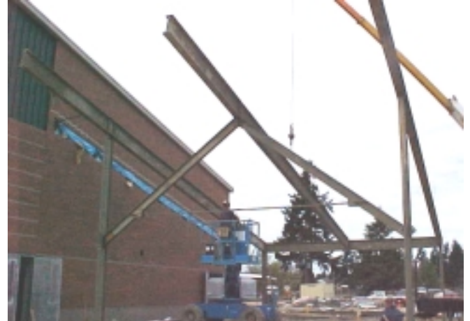
03/25/05 – North Hill Elementary - Looking North as covered play area is erected on east side of the Gymnasium.
